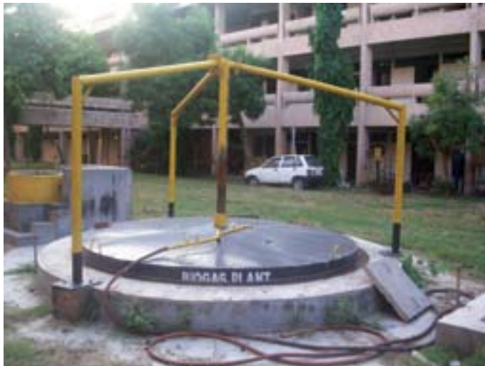
Figure 4a A pictorial view of 20 m 3 /day capacity floating drum biogas plant before start of feeding of de-oiled seed cake
