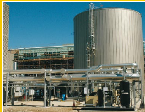
Industrial: Industrial site with CHP in northern Italy
