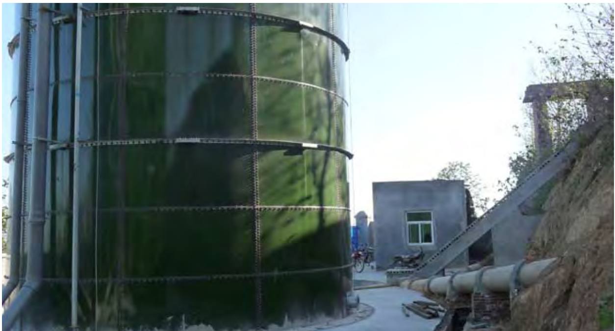
Biogas digester helps reduce emissions and provide clean energy in PRC, F. Radstake 2008.
