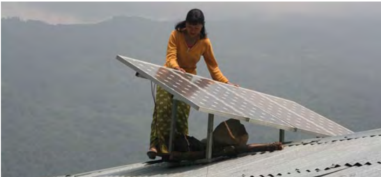
Solar installations provide clean, reliable energy to households, ADB Photo Library 2009
