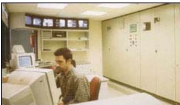
Monitoring System and Control Room
