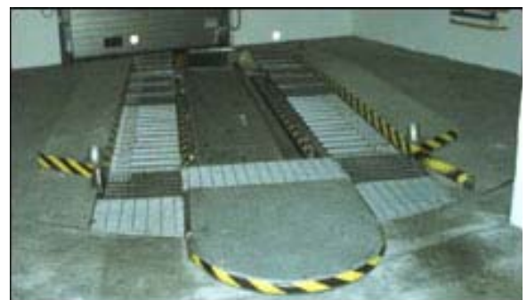
Entry Exit with Turntable
