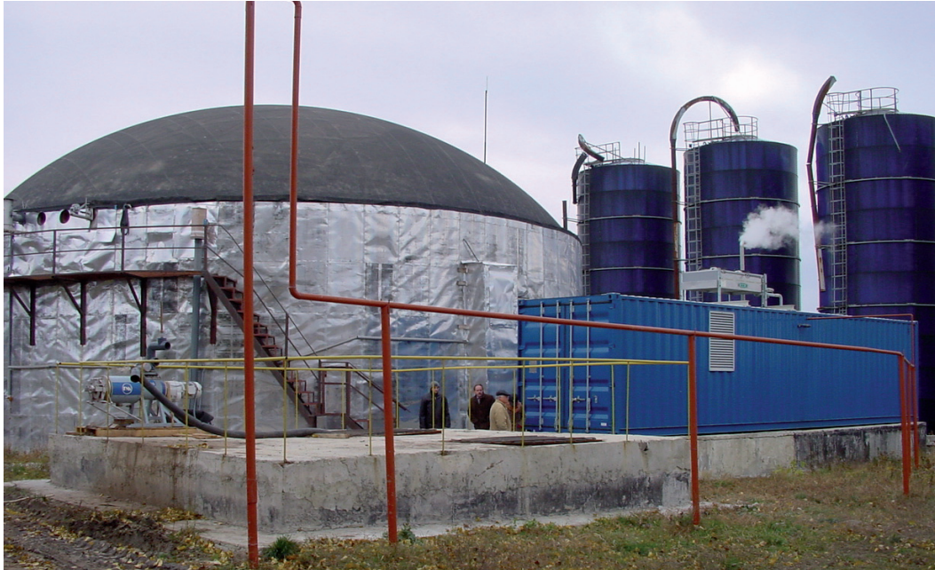
Figure III. Cow manure digester in Moldova
