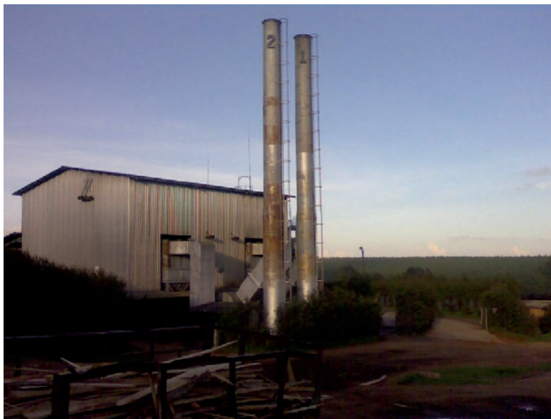
Figure XVIII. The TANWAT Power plant [67]
