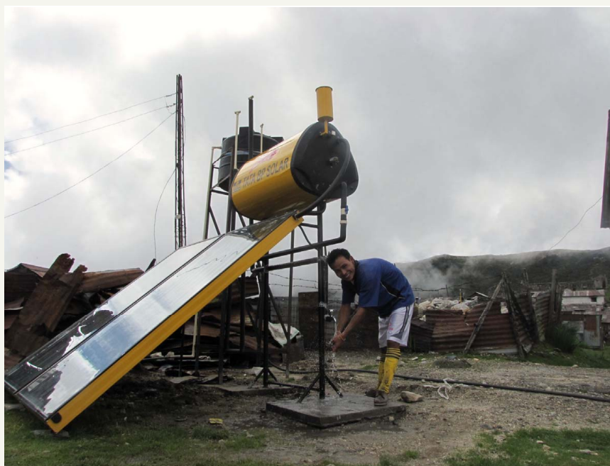
Solar Water Heater at Giathang village, East Sikkim District
