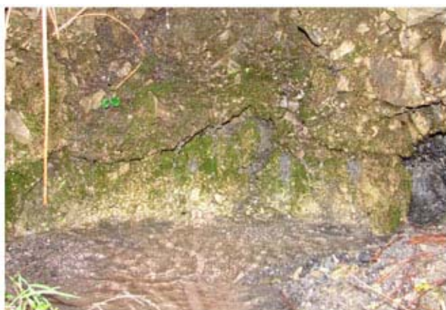
Figure 2. A view of seeping water from aquifer formation inside the tunnel.
