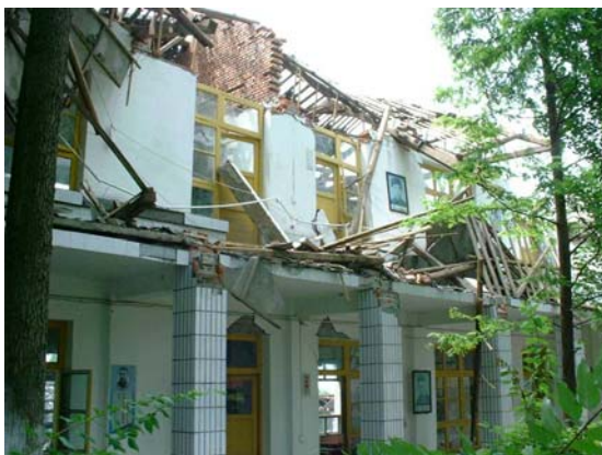
Figure 1.3 Damaged school building in Sichuan (June 2008)
