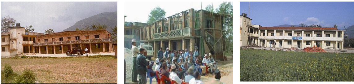
Figure 1.5 School Retrofitting in Nepal (2002): before - during - after (NSET) Discussion and observation of work were carried out during retrofitting.
