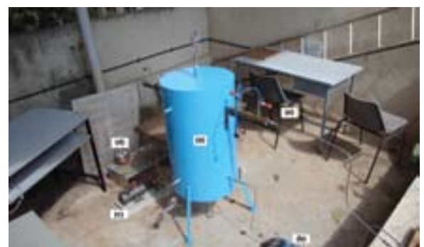
(a) buffer tank, (b) buffer-collector pump, (c) buffer-load pump, (d) heat exchanger, (e) flow meter
