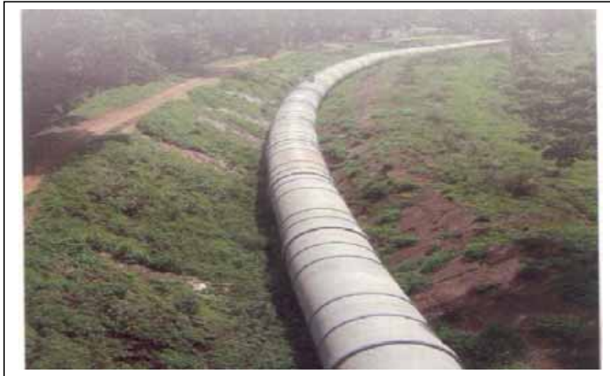
Plate 3.4 : Pipeline carrying Raw Water from Khadakwasla
