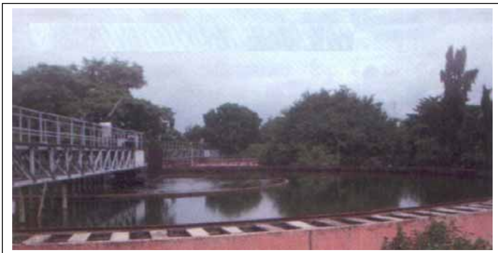
Plate 3.5 : Clariflocculator at Parvati Water Works
