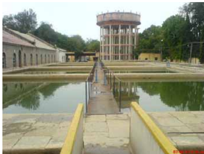
Figure 3: Sedimentation Basin and Elevated Service Reservoir at Asif Nagar Water Treatment Plant
