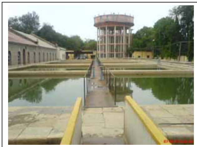
Plate 3.2 : Sedimentation tanks at Asifnagar Water Treatment Plant
