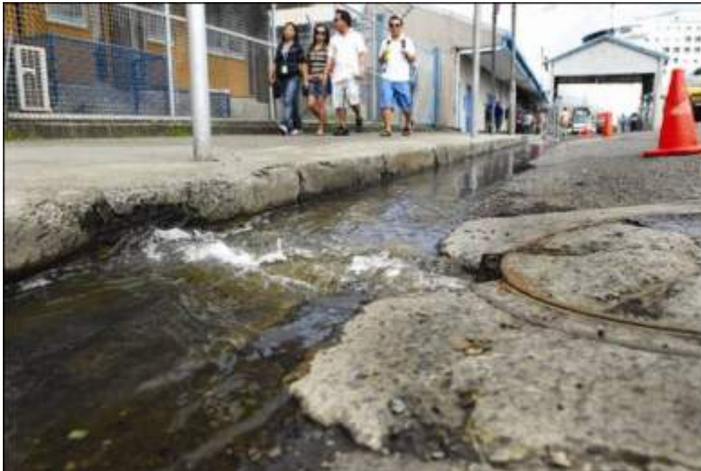
Plate 2: Overflowing Sewage in front of Fiji Ports Corporation Limited head office at the Kings Wharf in Suva. (The Fiji Times – 16 October, 2008).
