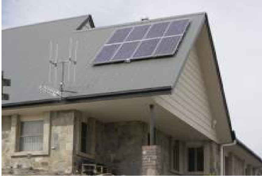
Solar panels ©DEWHA
