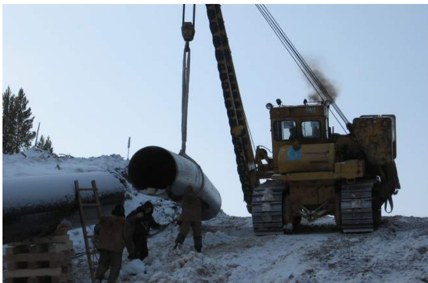
Pipeline construction on the Northern Amurskaya Oblast (Tynda District) Photo by Tatiana Tonkikh (Tynda)
