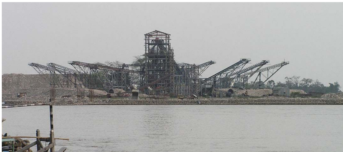
Fig-28: Ongoing construction of water development project on Subansiri River at Garukamukh
