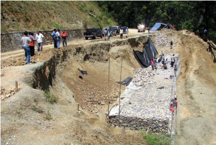
Adaptation to climate change is key component in infrastructure development by strengthening engineering design of a road construction
