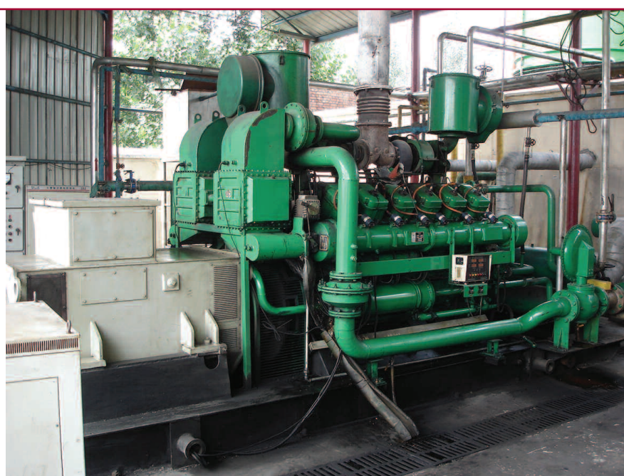
FIGURE 9: LOW GAS QUALITY 500KW SHENGDONG ENGINE
