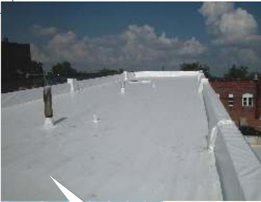
Insulate the roof with materials such as rock wool, mineral wool, EPS, XPS, vermiculite, and so on.
