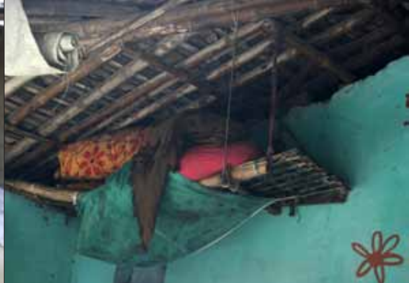
Figure 18: Construction of Machhan below the roof for storage and protection of valuables during floods
