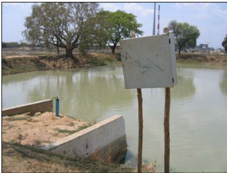
A water pump has been installed in Patadi but has yet to be wired up and so cannot be used
