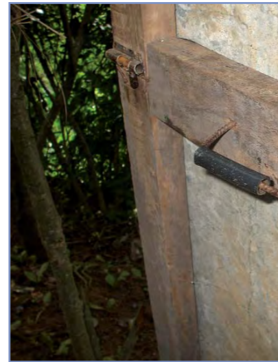
Photo 15: Handle of rod and pipe to make it easier to pull door closed from inside
