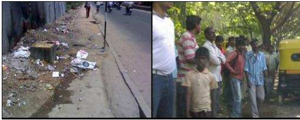
Figure 1 & 2 indicates sorry state of footpath (not in proper shape and not sufficient)
