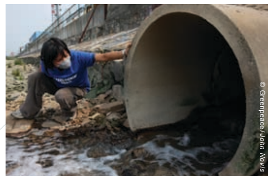
A discharge outfall connected to the outside wall of the industrial area
