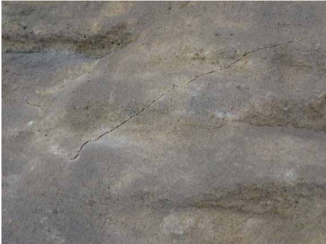
Figure 37: Minor Cracking (Exfoliation) in Rock Shelter Wall, Ousedale Creek, October 2007
