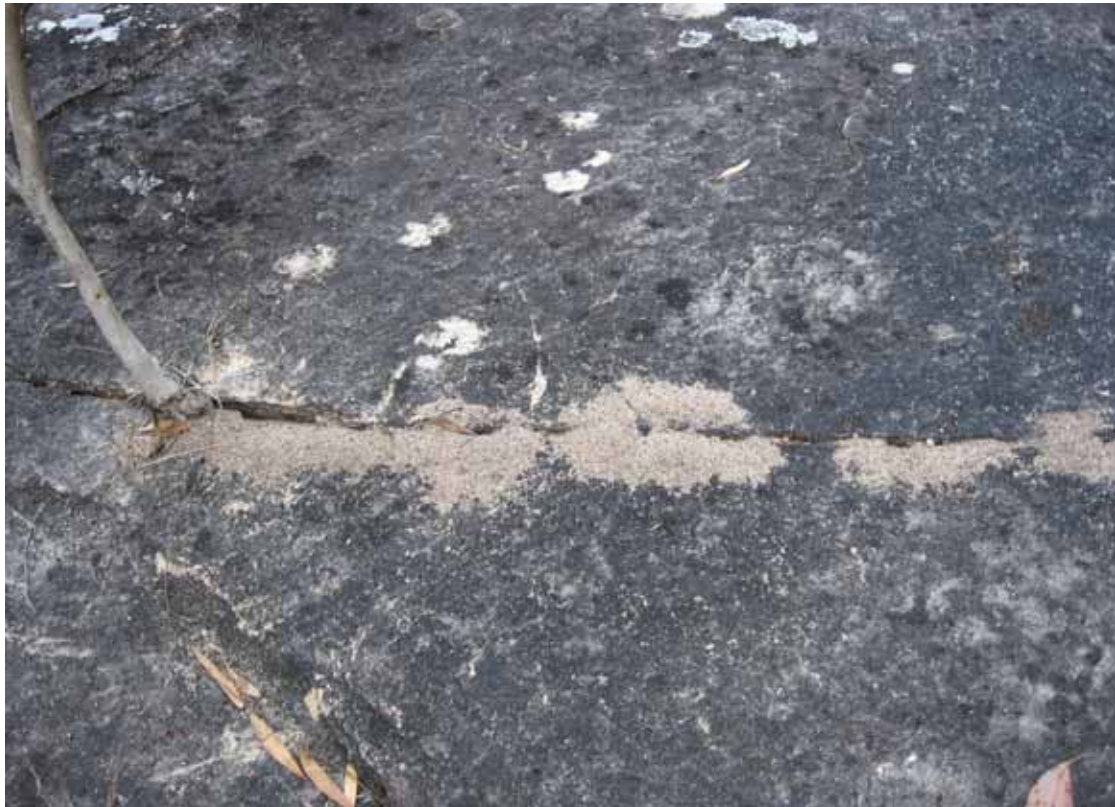
Figure 41: Colonisation of Subsidence Crack by Sapling and an Ant Nest, Lower Cataract River, September 2007
