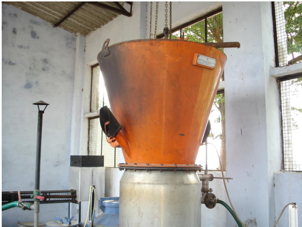
Photo 2.6: Biomass Gasifier installed at Shri Nagar
