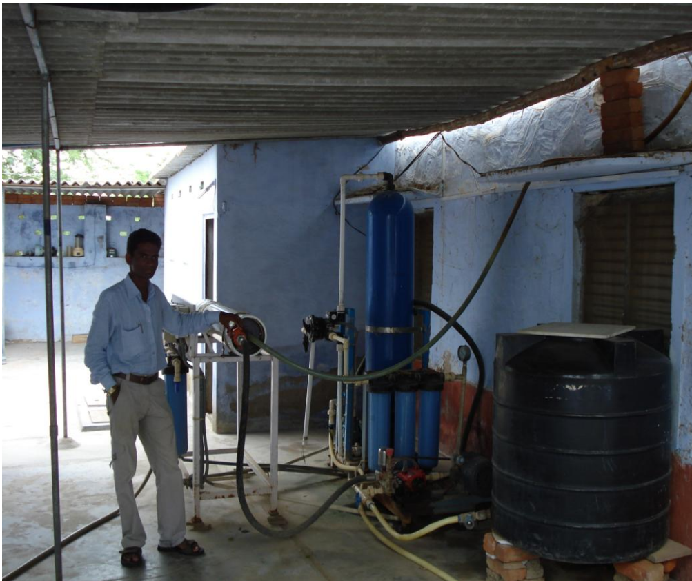
Photo 4.4: Reverse Osmosis Plant at Kotri
