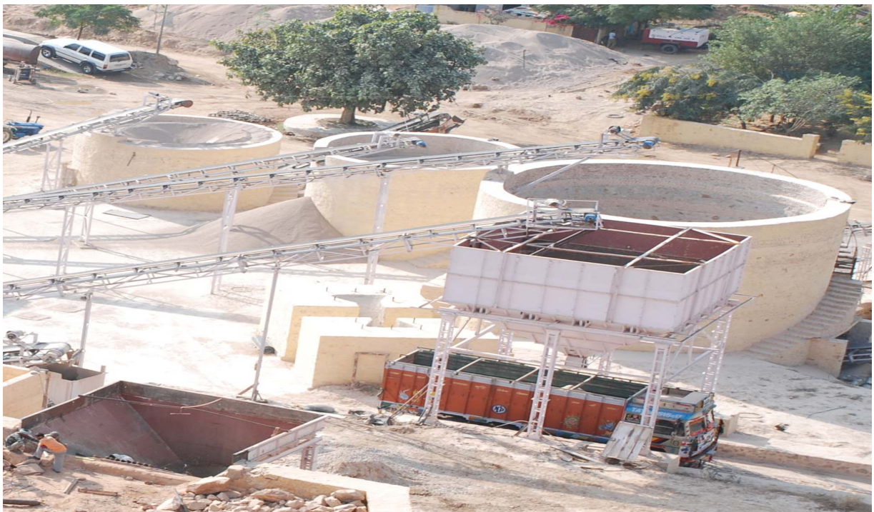
View of the hoppers for the material & dust collection
