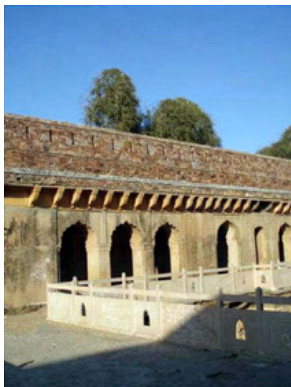
Baawri - under attack of vandalism, Neemerana
