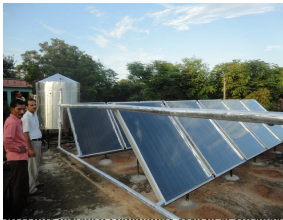
Figure 16.1 Recently installed community system at Piranagar, Dist Kathua, J&K
