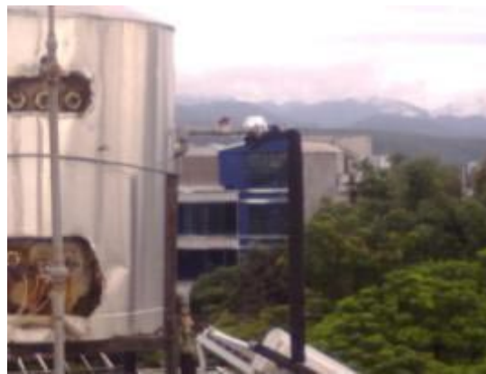
Lack of proper insulation on the solar tank
