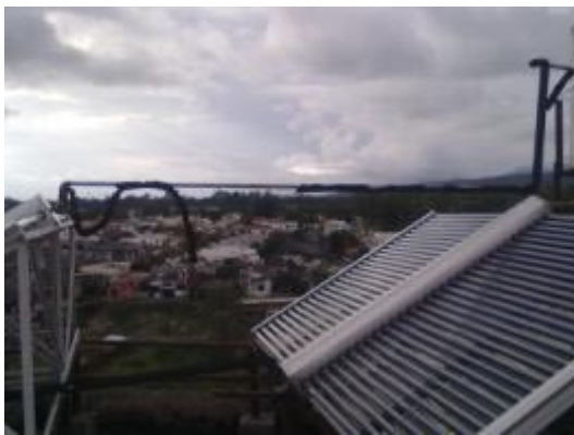
Rubber pipe insulation in Hotel Maggi star
