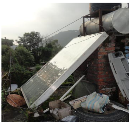
Fig 16.3: A 15 yr old Residential SWH installation in village Guggar (Dharamsala – Palampur Road)
