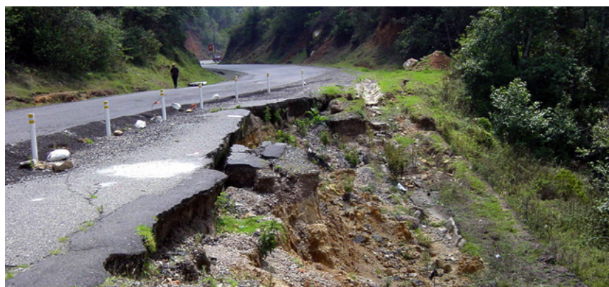
Figure 10 Flood damaged road in Guatemala.
